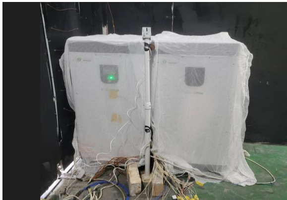
Fig 3 BESS Test Setup
